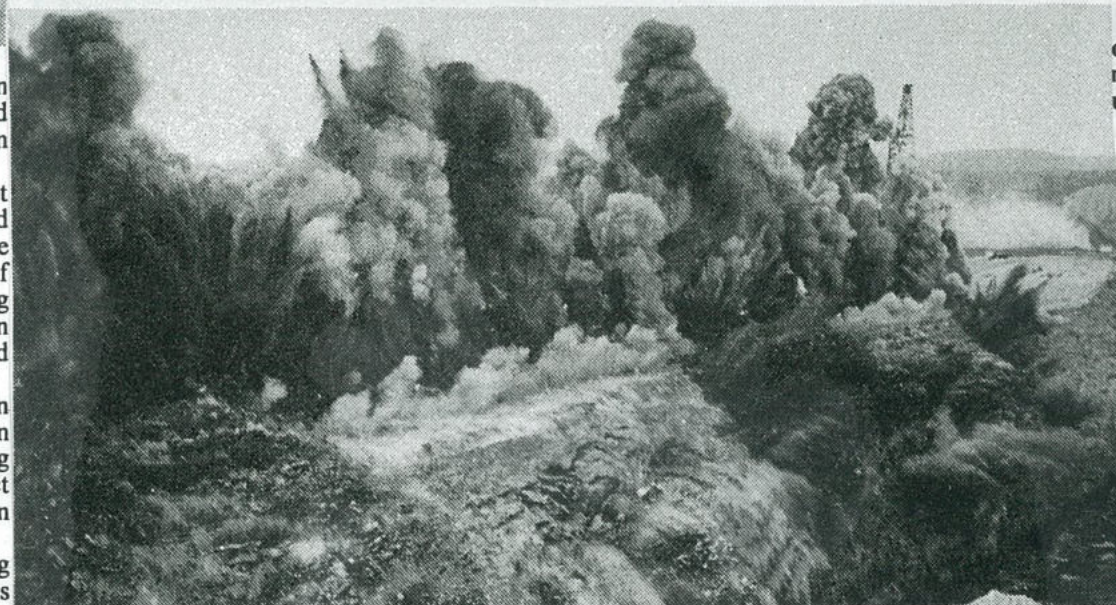
The plumes fuse into clouds of rock and soil leaving only the boom visible . . .
